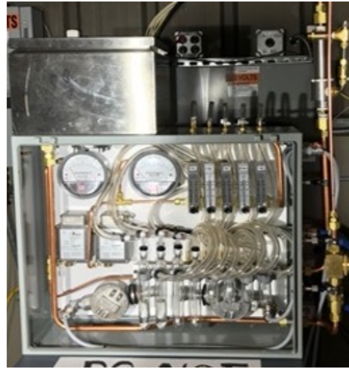
Gas Distribution Panel
