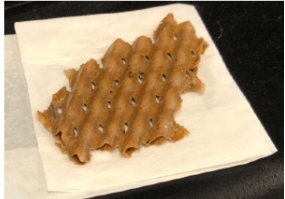
Gunk stuck in the heat exchanger
