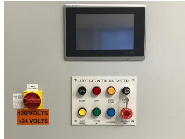
Front of the controls cabinet
